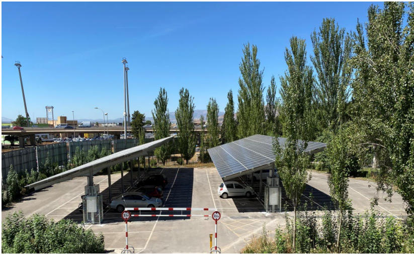
Image source: Owned by DPG partner. PV facilities in its parking lot.
