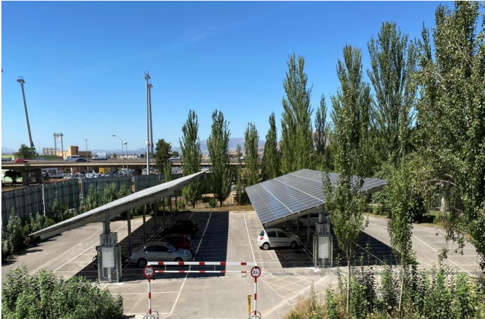
Source: Owned by DPG partner. PV facilities in its parking lot.
